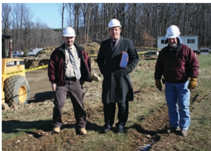
(From left to right) PWCampbell Construction Management, Project Manager, Michael Schaupp, Picatinny Federal Credit Union President & CEO, Bill Darling and Site Project Manager, Bill Taylor review the progress of the new Mt. Olive Branch location at a weekly construction meeting.
